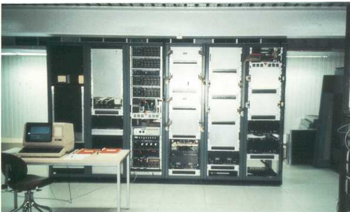
Back-ends installed in the equipment room on the Plateau de Bure.
