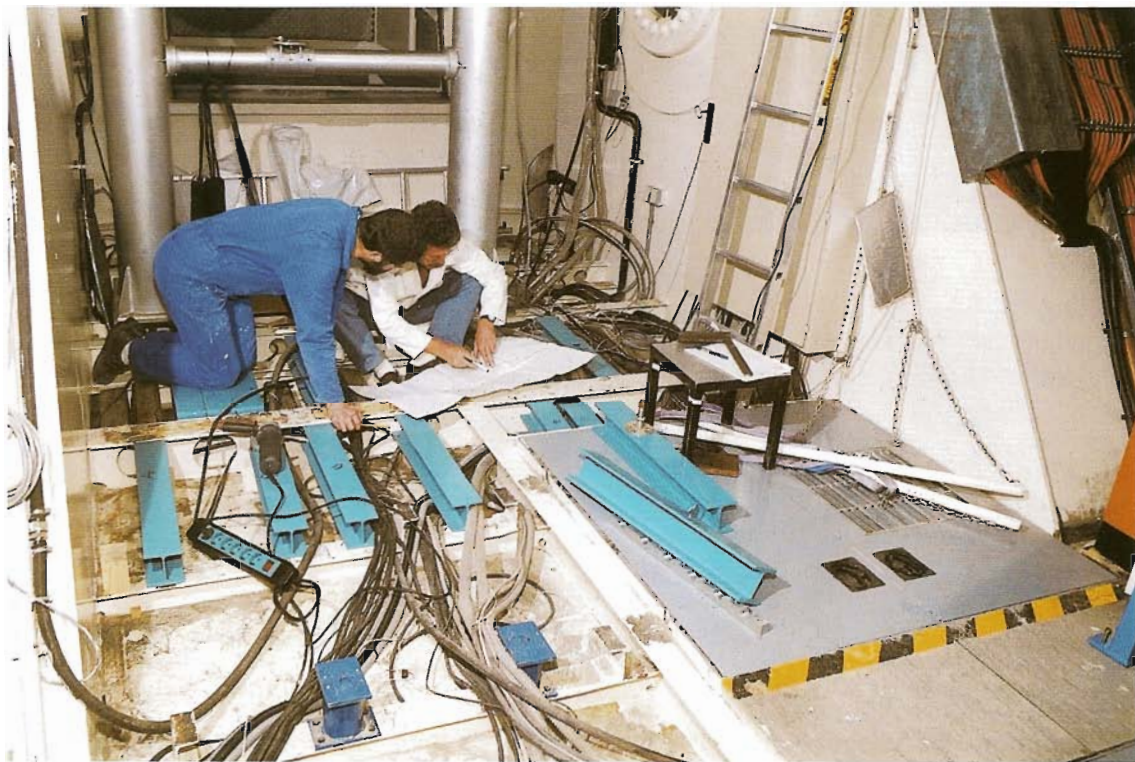
Fig. 3.6: Work in the receiver cabin. The floor is prepared for the new receiver support structure.
