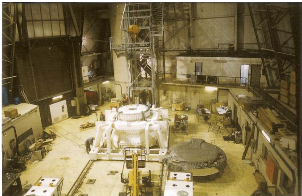
Fig. 4.3: The beginning of the assembly work for Antenna 6 on the Plateau de Bure.
