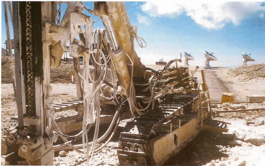
Fig. 4.4: A drilling rig close to N29 during the preparation of the ground levelling work for the new track extension. Far in the background three antennas of the interferometers kept at a safe distance from the blasting areas.
