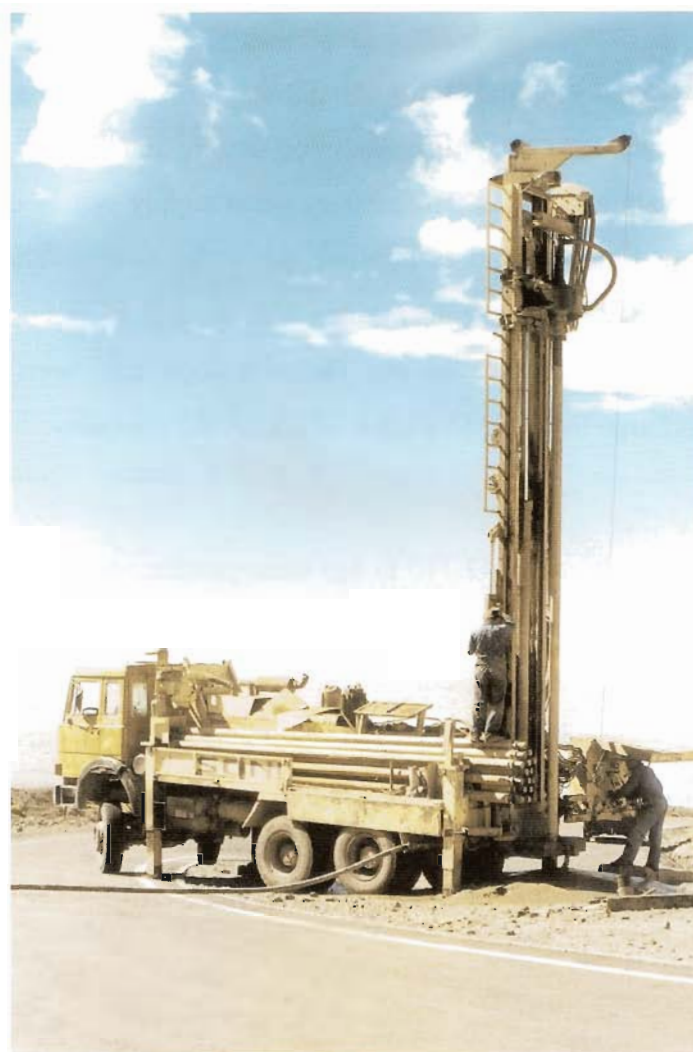
Fig. 3.8: A 40 m deep hole has been drilled into the rocky soil to provide a new electrical grounding of only 2 ohms.
