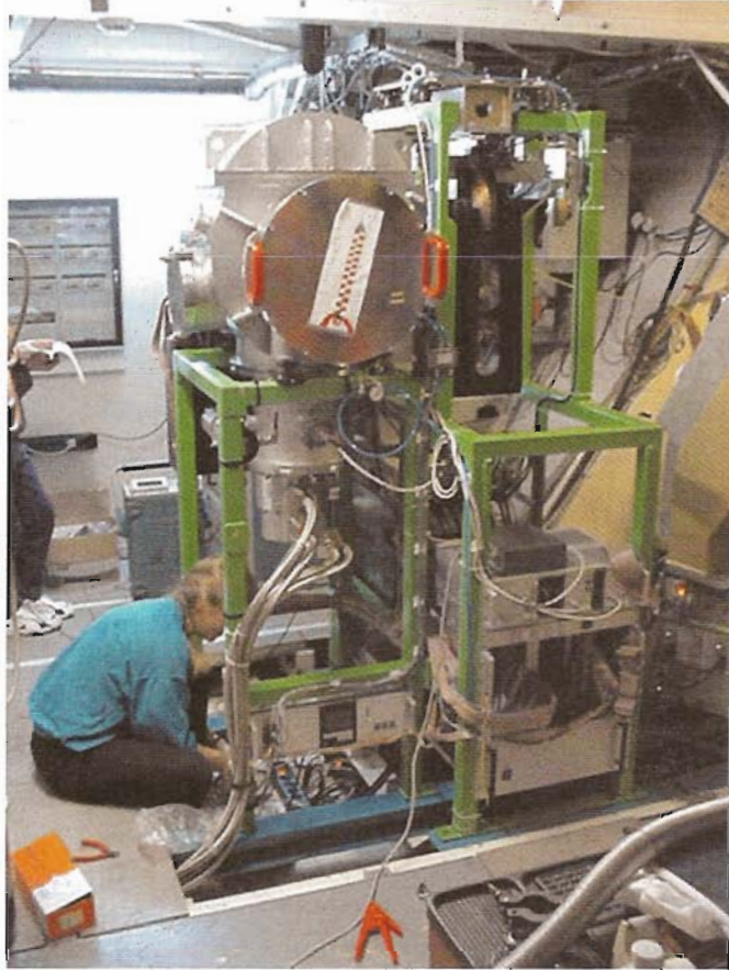
Fig. 5.3: HERA at the 30m telescope during the final phase of installation and cabling in May 2001. The whole system is self contained including cryogenics, RF and control electronics in order to minimize space requirements in the 30m cabin. To the right of the stainless steel cryostat the the K-mirror of the derotator unit is visible (black).
