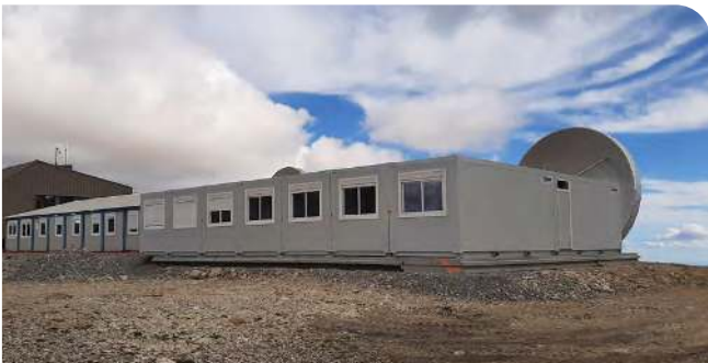
Top: Additional living quarters for personnel of the building site et relaxation area.
