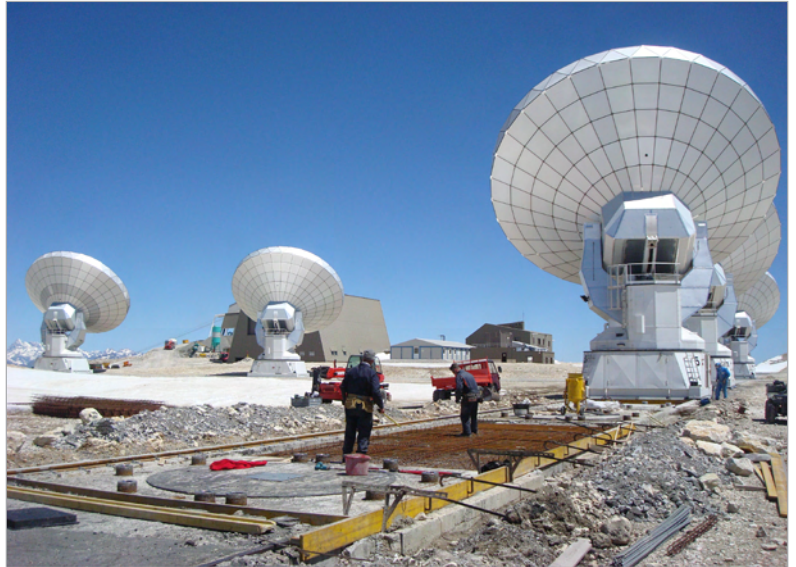
Sidetrack construction and pavement refurbishment work on the western track, as of June 05, 2012.
