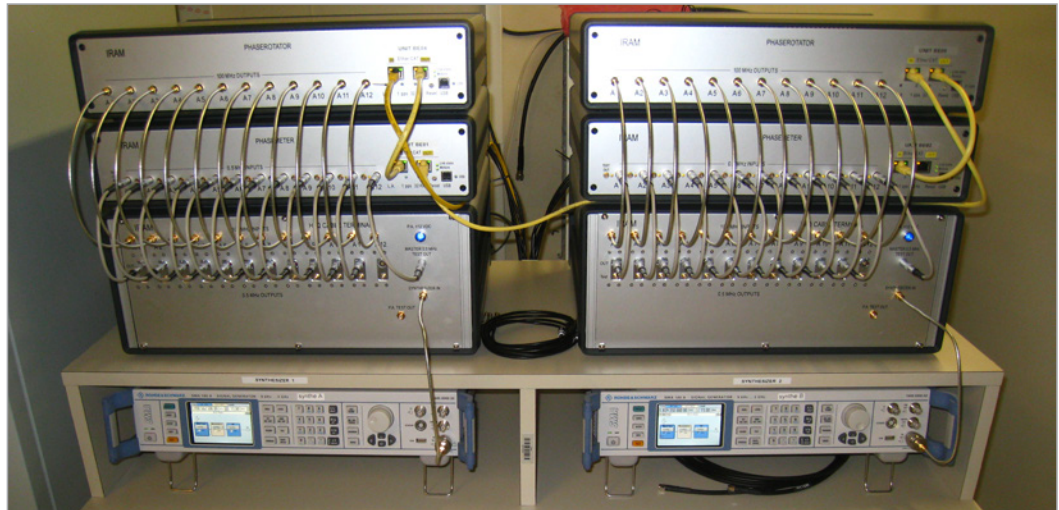
Low phase noise LO reference system for 12 antennas in operation on Plateau de Bure
