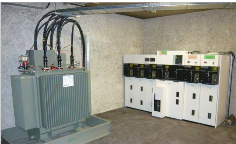
New high voltage transformer and cell of the extended power supply system of NOEMA.
