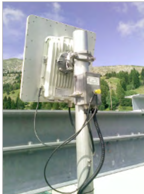
The new WIFI antenna near the NOEMA lower cable car station.
