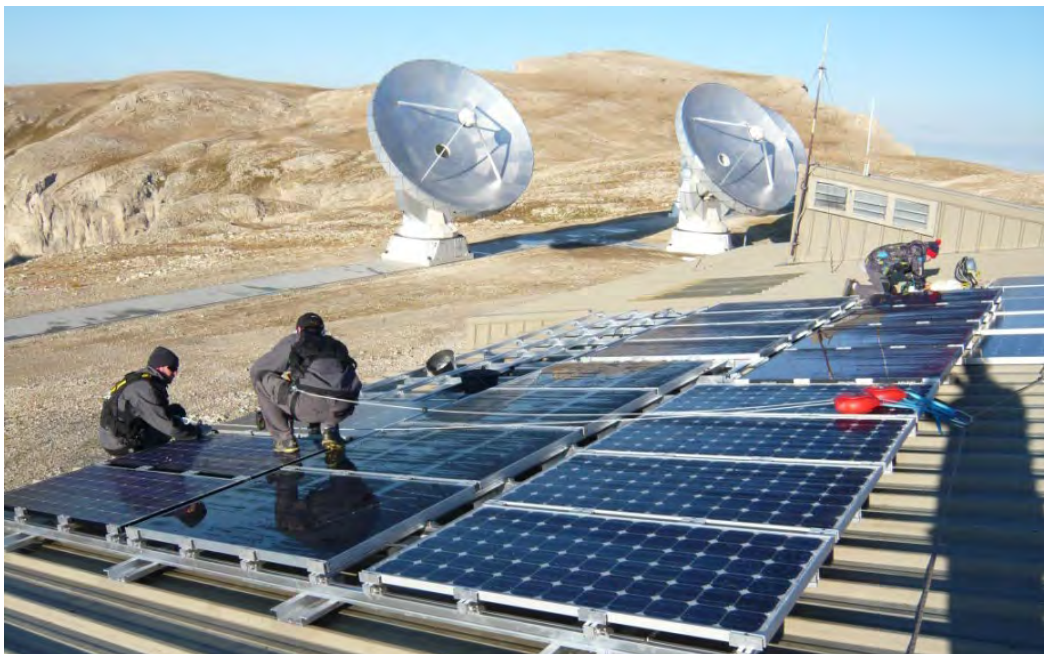
Installation of solar panels for the INES experiment on the observatory main building.
