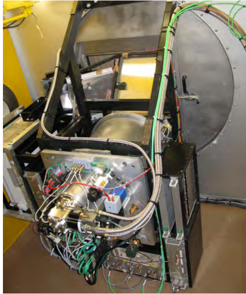
NOEMA receiver during its lift-off into an antenna (left) and after installation in the receiver cabin (right).
