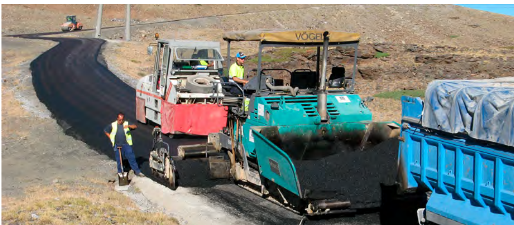
Work on the upper access road to the 30-meter telescope in August 2015.
