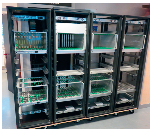
View of the 4 cabinets partially populated with future racks.
