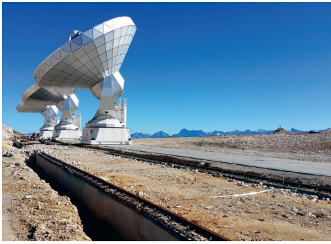
Top: NOEMA antennas performing science observations during the construction of the northern bypass track.
