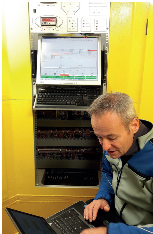
NOEMA engineer performing a system verification review in the pedestal of antenna 9.
