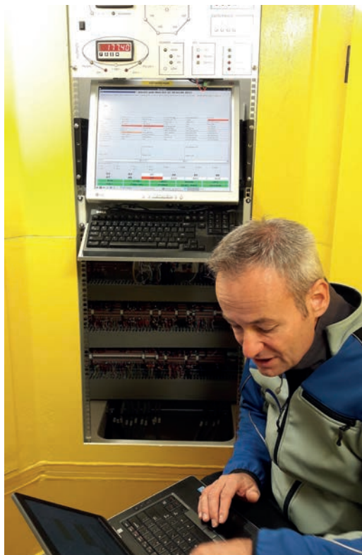
NOEMA engineer performing a system verification review in the pedestal of antenna 9.
