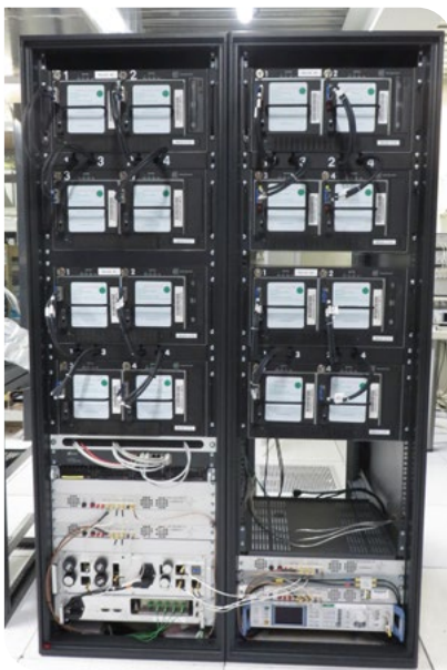
VLBI Mark 6 recorders installed at NOEMA.
