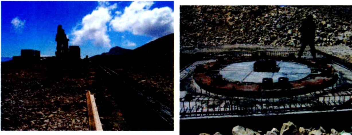
Fig. 4.14: On the left: Form working and casting of a portion of the southern track support of the Eastern track extension. On the right: implementation and control of the location of the centring ring of the station N46.
