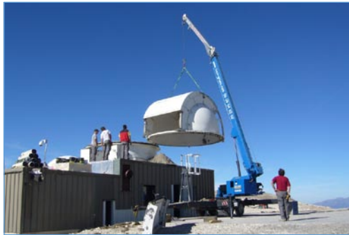
The dismantling of the dome of POM2 on the Plateau de Bure
